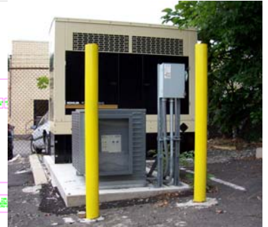
New Emergency Generator
