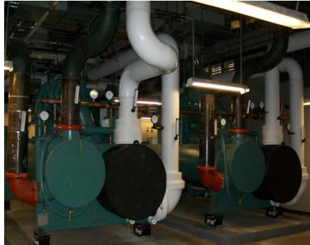
Variable Flow Chillers
