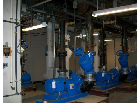
Chilled Water & Condenser Water Pumps
