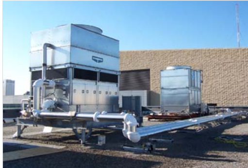
New Evaporative Cooler & Cooling Tower
