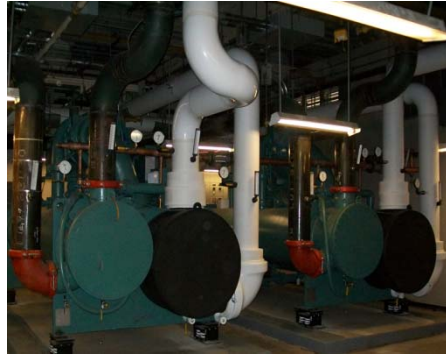
Variable Flow Chillers
