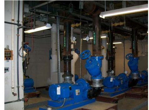
Chilled Water & Condenser Water Pumps
