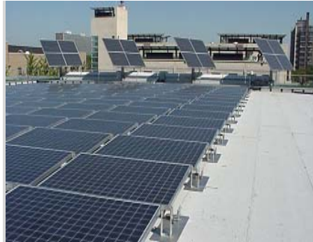
PV Array and Tracking Modules
