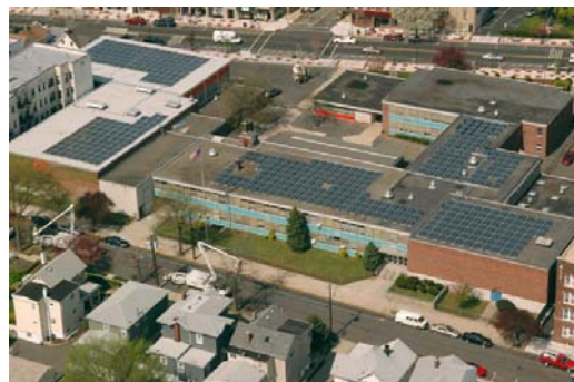
207KW Photovoltaic Array at Lincoln School
