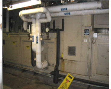
Cargo-Care AC Unit
