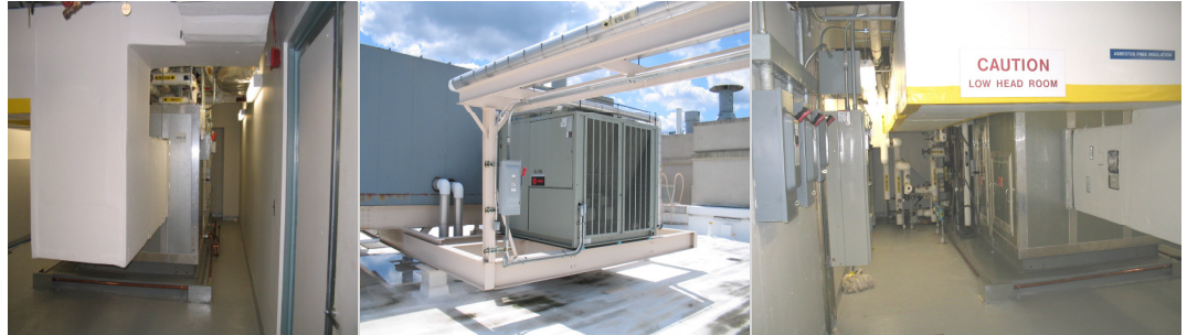
Air Handling Unit
