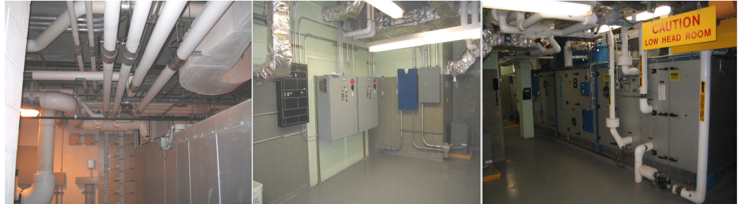
Chilled and Hot Water Piping
