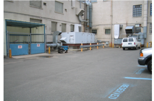
Air Conditioning Unit for PNU Expansion
